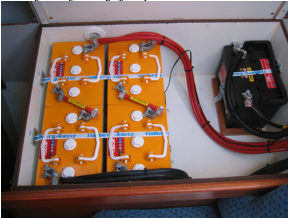
A professional battery installation: starter battery in black (to the right) and deep-cycle batteries in yellow (to the left). Foto: Marcus Åkesson
