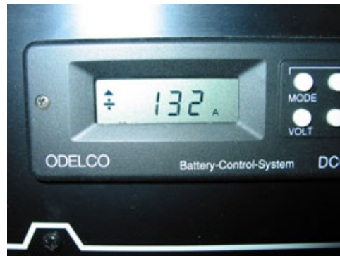
With new cables installed and we receive over 130A during bulk charge, compared to some 90A with the thinner cables.
