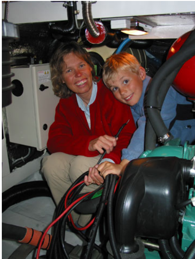
Karolina and Jonathan in the engine room working with exchanging the feeder cables
