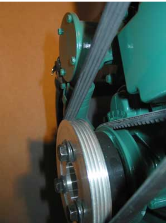
Volvo uses a single belt with 4 "Vs" to transmit the 2.2 kW from the engine to the 220V alternator
