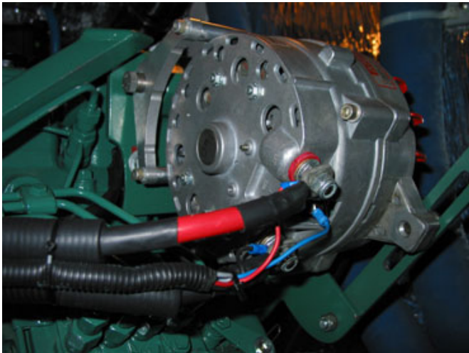
The new 50 mm 2 feeder cables fitted on the alternator. The smaller cables are control cables from the regulator.
